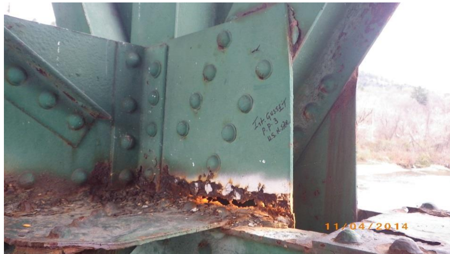
Figure 4: Example of Steel Deterioration on a Municipal-Owned Bridge
