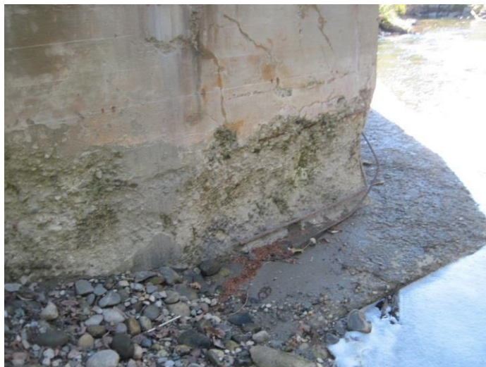
Figure 6: Example of Effect of Scour on a Municipal-Owned Bridge
