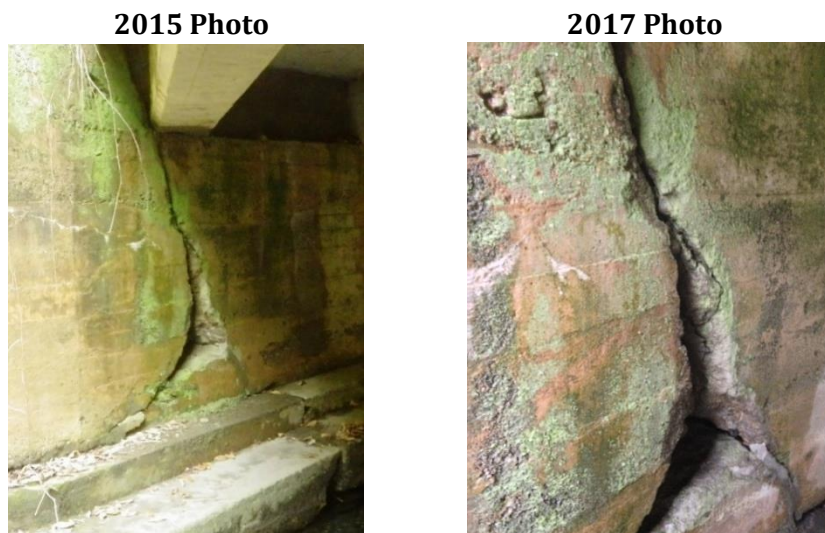
Figure 8: Crack in Randolph Bridge #36 Abutment
