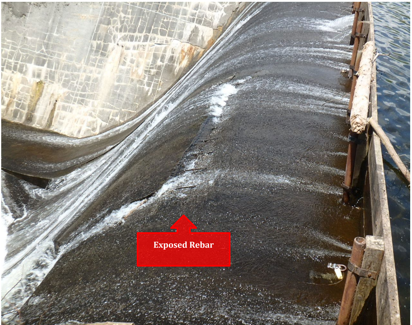
Figure 6: Exposed Rebar in the Thurman W. Dix Reservoir Dam in Orange, Vermont
