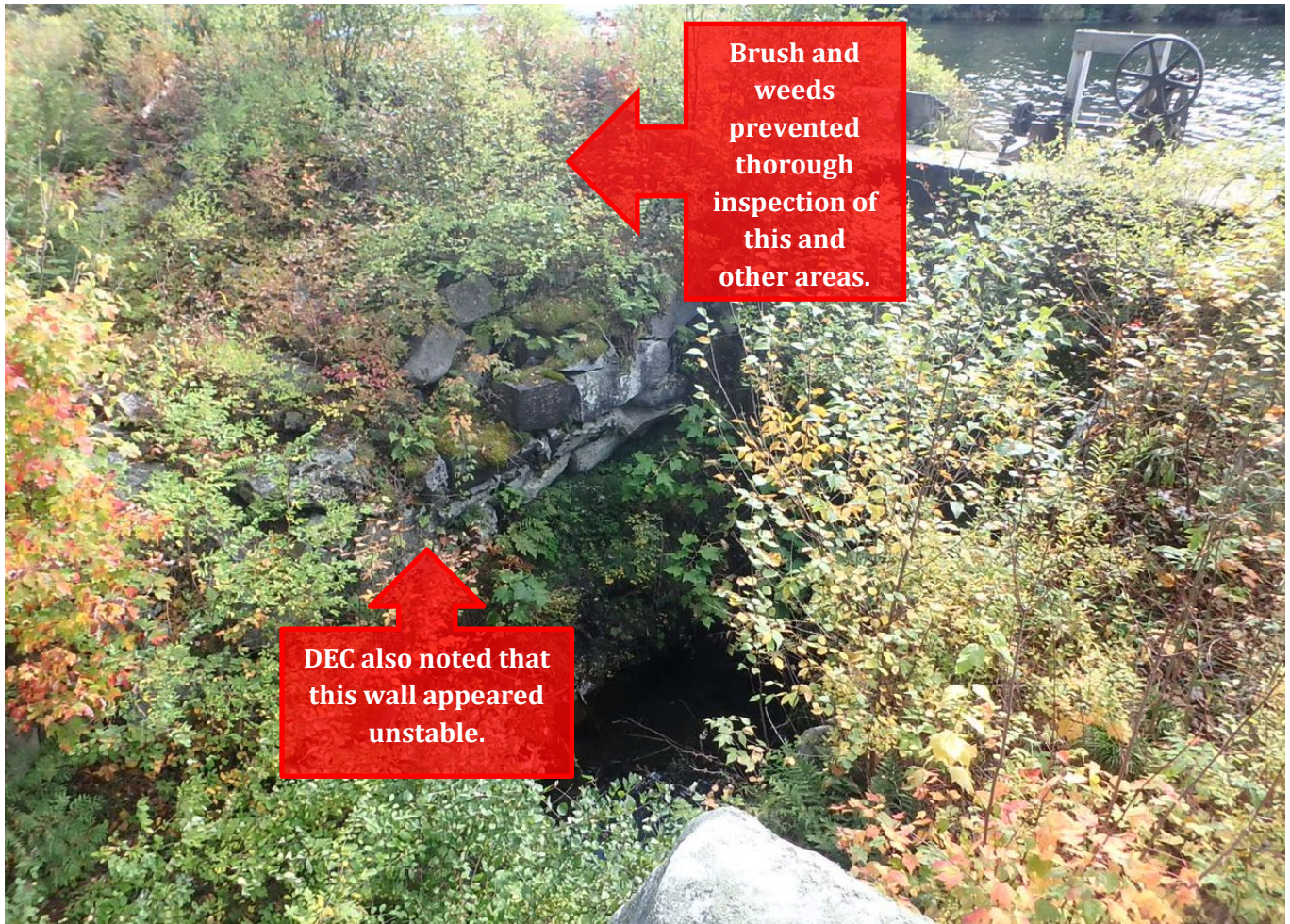
Figure 7: Brush and Weeds Around a Portion of East Long Pond Dam in Woodbury, Vermont a
