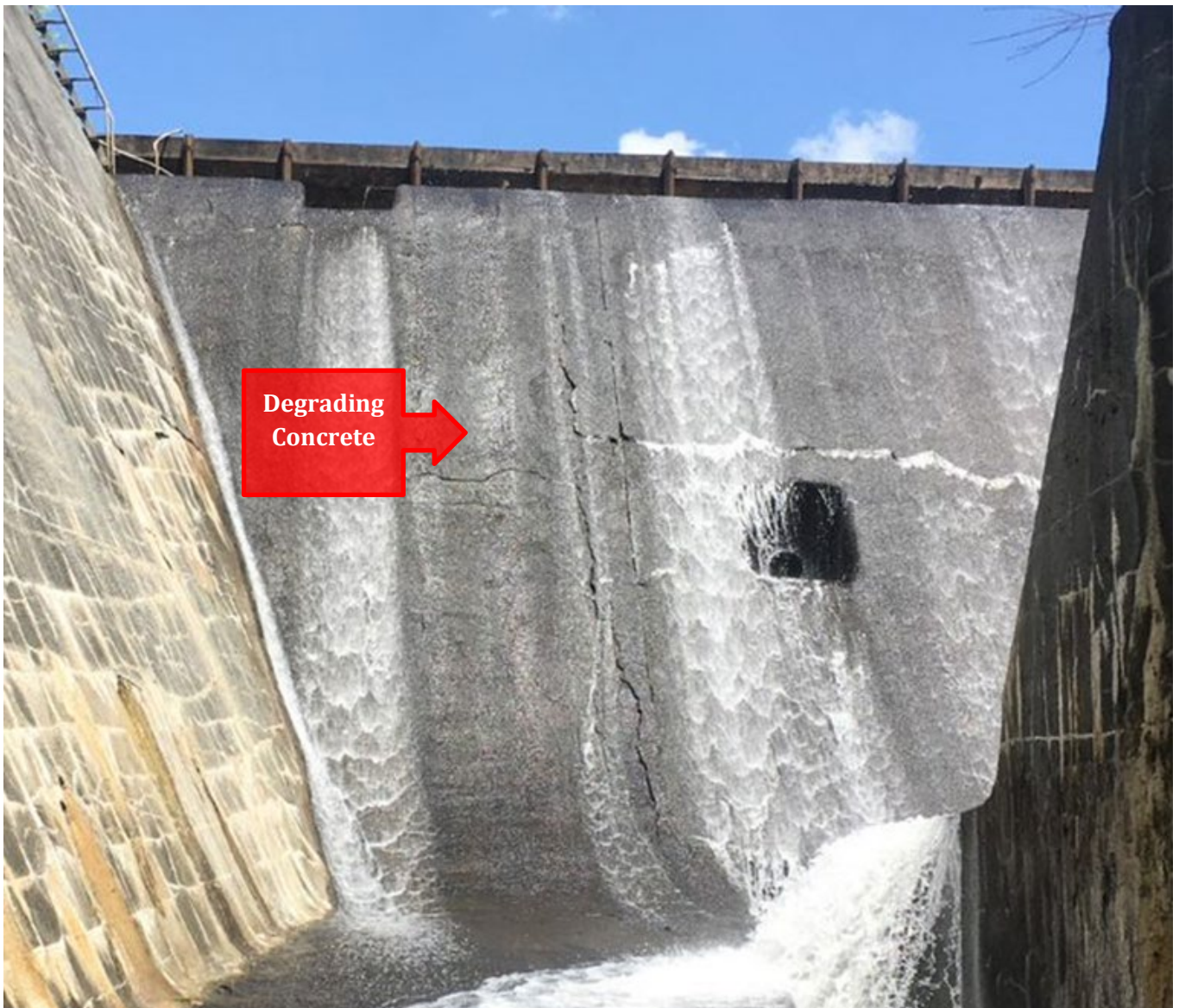
Figure 5: Degraded Spillway in the Thurman W. Dix Reservoir Dam in Orange, Vermont
